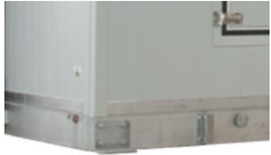
Compact Substation Base
