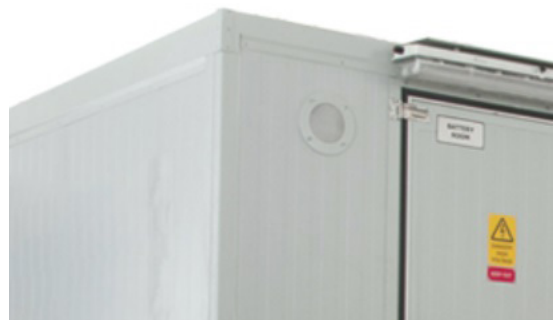
Compact Substation Roof
