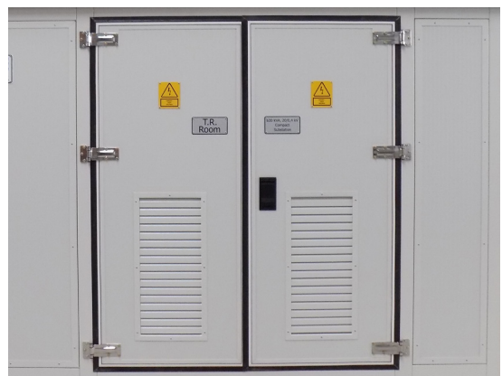
Compact Substation Door
